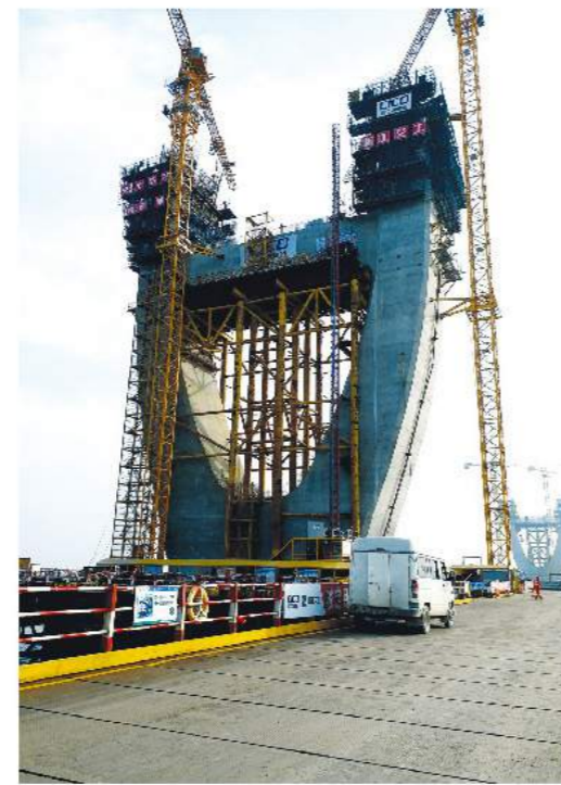
Project name: Section 1, 2, 3 of the main channel of Zhoushan Port, Ningbo Contractor: Zhejiang Jiaogong Group Co., Ltd. CSCEC China Communications Road and Bridge Construction Co., Ltd. Products utilized: ACS, HCB-100 (Separate Truss Type)
