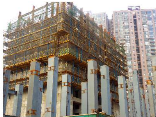
Project name: Harmonious Century Square Contractor: Yunnan Jiangdong Group Construction Engineering Co., Ltd. First Engineering Office Products utilized: ACS, HCB-100 (Separate Truss Type)
