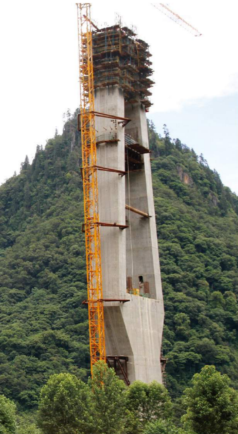
Project name: Polonggou Bridge Contractor: China Railway Bridge Corporation Products utilized: ACS, HCB-100 (Composite Truss Type)
